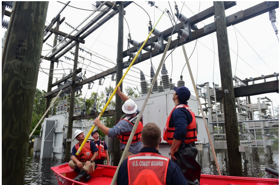
U.S. Coast Guard members escorted utility workers to perform repairs on transformers at a flooded substation in Newport, N.C. | U.S. Coast Guard
